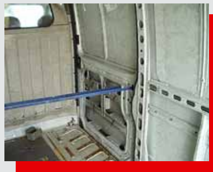
Parts that have been kept in place through emergency repair or do not serve their original function any longer. Missing interior lining or partition walls.
