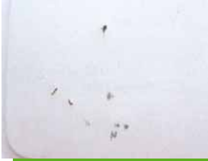
Damages in paint not through to basic material.
