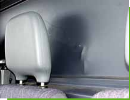
The partition wall shows dents but is not influenced in its function.
